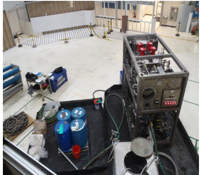
Process Equipment Setup at Press 12
