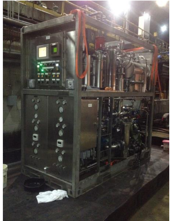
IAS 2135 Advanced Fluid Purification Skid staged at the Twist Mill oil reservoir. Used to decontaminate and purify Shell Morlina 100.
